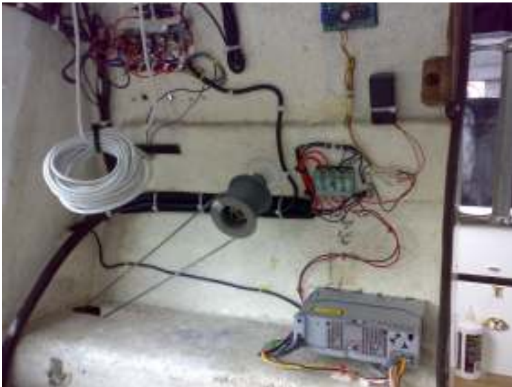
This shows CD player, bottom right, mounted. (Please excuse unfinished wiring) from inside cabin.
